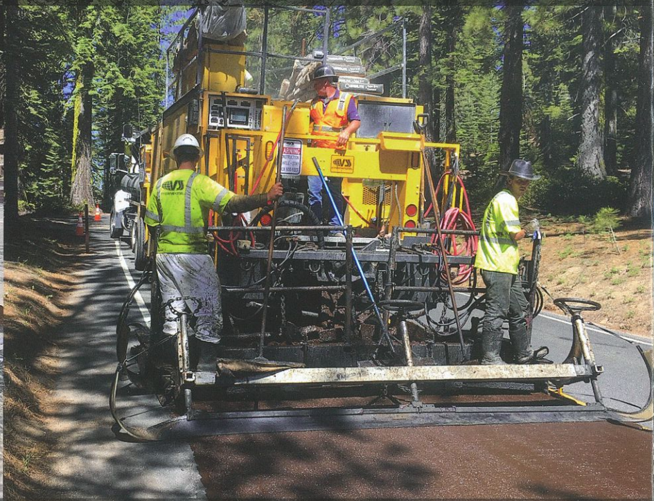
Mainline application of microsurfacing at Tioga Road near Tamarack Flat Campground - elevation 7,042 feet.
