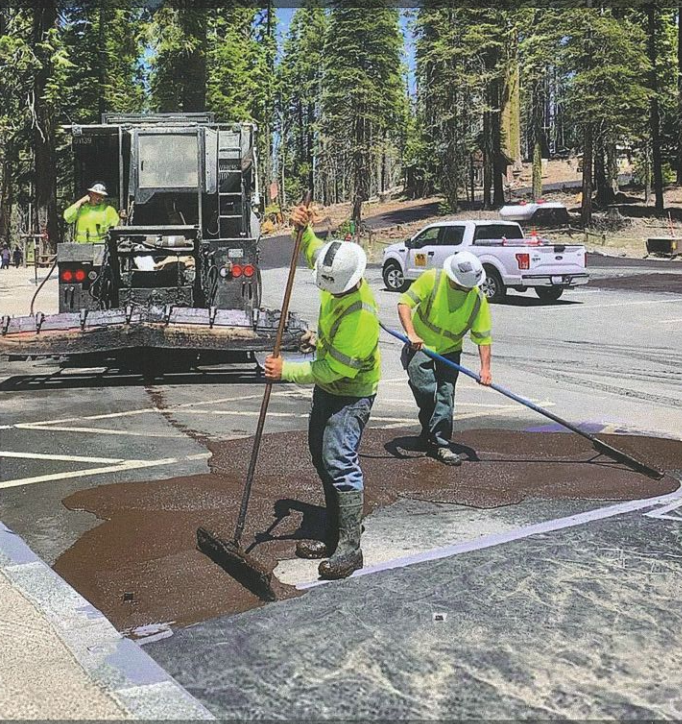
Keeping granite curbs clean required attention to detail while performing hand work at Tuolumne Grove Parking Lot - elevation 6,195 feet.
