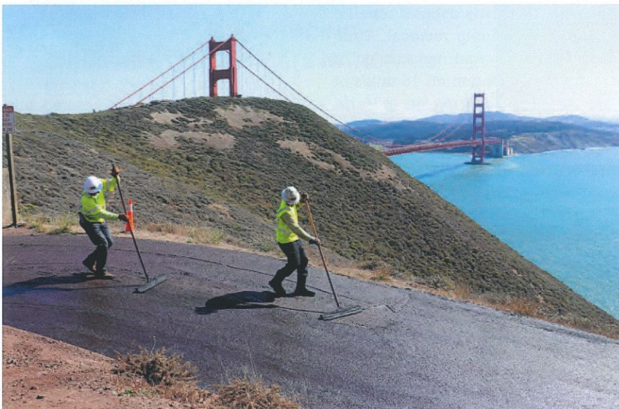
A mixture of aggregate and ambient temperature asphalt emulsion, micro surfacing is designed to adhere to the asphalt concrete surface
