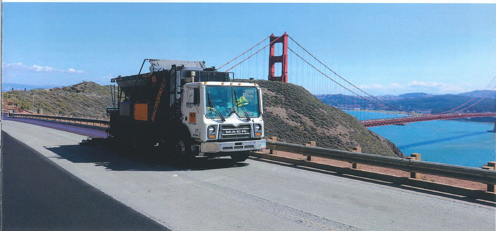
Specialized applicator truck places micro surfacing on grade in Golden Gate National Recreation Area above the Golden Gate to San Francisco Bay and San Pedro Bay
